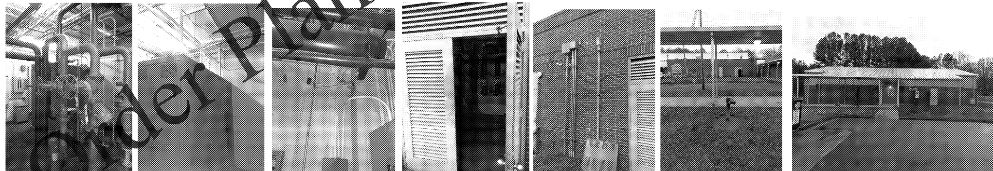
EXISTING MAIN SWITCHBOARD LOCATED IN BOILER ROOM. EXISTING MAIN SWITCHBOARD. EXISTING INTERIOR WALL OF BOILER ROOM. EXISTING EXTERIOR DOOR TO BOILER ROOM. EXISTING EXTERIOR WALL OF BOILER ROOM. VANTAGE POINT STANDING NEXT TO MULTI-PURPOSE BUILDING LOOKING AT BOILER ROOM. EXISTING MULTI-PURPOSE BUILDING.
