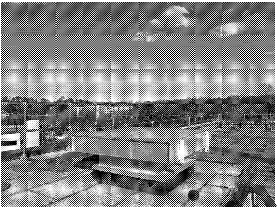
A PICTURE (EXISTING CONDITIONS, FOR REFERENCE ONLY) NTS NOTE: EXISTING HOIST WAY VENT TO BE DEMOLISHED AND REPLACED WITH NEW. REFER TO DETAIL 3/MH601 FOR NEW HOIST WAY VENT AND FLASHING REQUIREMENTS.
