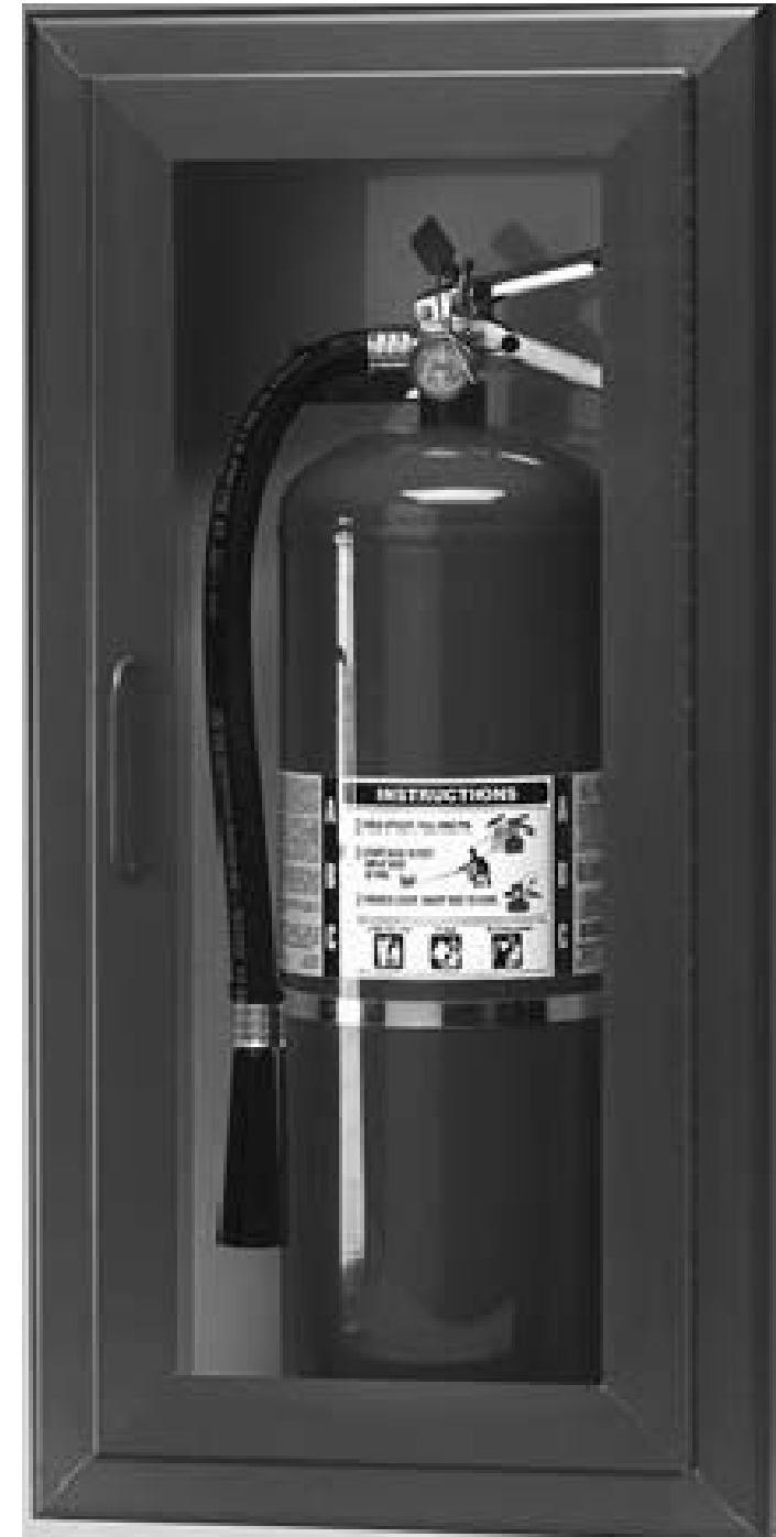
INSTALLED FINAL LOCATIONS AND QUANTITIES BY FIRE MARSHALL.
